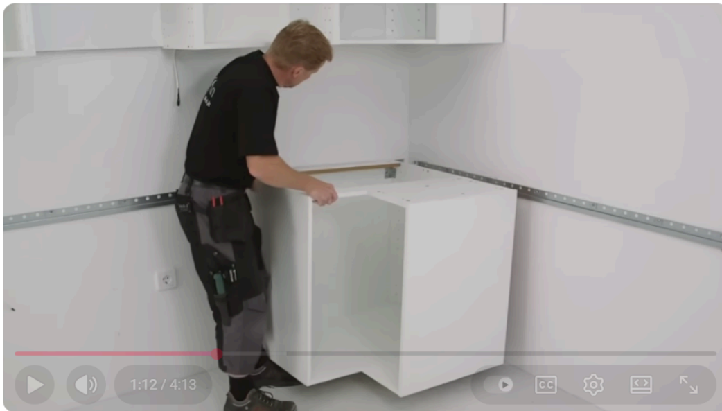
Figure 3b: Installing IKEA kitchen cabinets on a wall-mounted steel cleat. Screen-shot from IKEA METOD Kitchen Installation 3/7 - Installing the cabinets.
